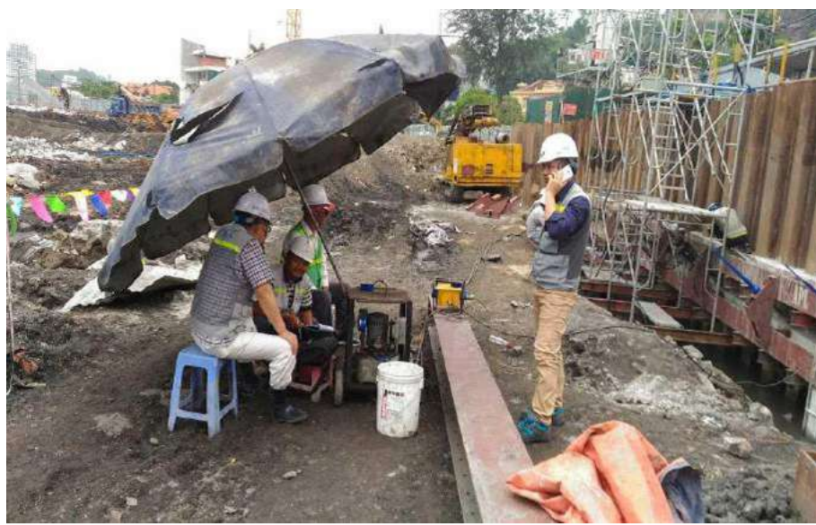
I supervise and accept for stress the Prestress Ground anchor of KRVINA subcontractor - Korea.
